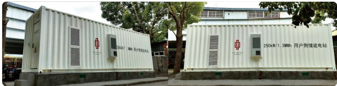
Application: CE -- 2501300 Time: December, 2021 Address: Ningbo, China Capacity: 250kW/1.3MWh
