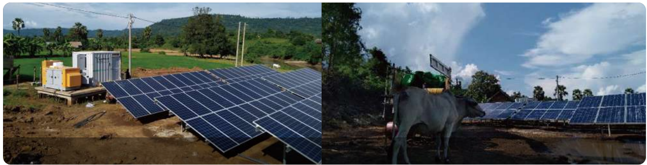
Application: Inverter -- CE0050 Solar Panel -- CE450-36V-MH Battery -- CE76120-160 Time: October, 2021 Address: Myanmar Capacity: 60kW/160kWh
