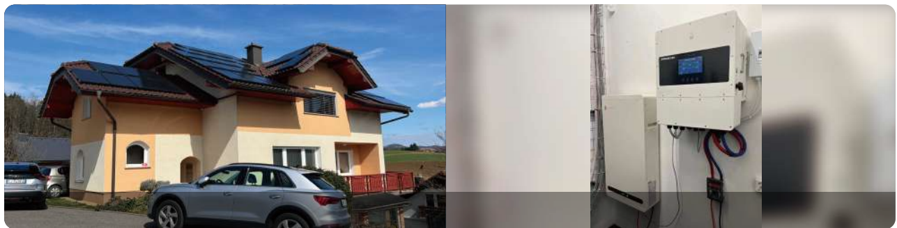
Application: Inverter -- Mars-12G1-LE Solar Panel -- CE410-27V-MH Time: June, 2023 Address: South Africa Capacity: 12kW/10kWh
