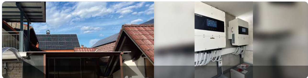
Application: Inverter -- Mars-12G1-LE Solar Panel -- CE410-27V-MH Time: May, 2023 Address: Lebanon Capacity: 12kW/10kWh
