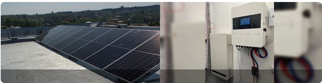
Application: Inverter -- Mars-12G1-LE Solar Panel -- CE410-27V-MH Time: Jun, 2023 Address: South Africa Capacity: 12kW/10kWh
