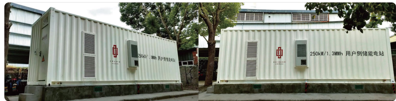
Application: CE -- 2501300 Time: Dec, 2021 Address: Ningbo, China Capacity: 250kW/1.3MWh
