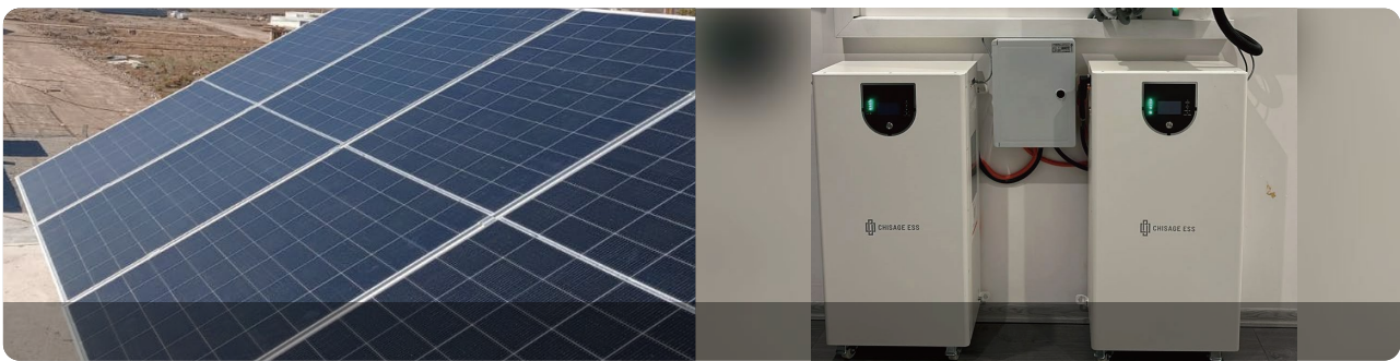
Application: Solar Panel -- CE410-27V-MH Battery -- MOON16-G Time: Oct, 2024 Address: Yemen Capacity: 6kW/32KWh
