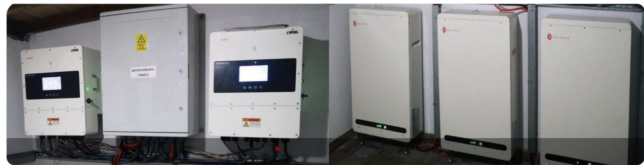
Application: Inverter -- Mars-12G1-LE Battery -- CE48200-W Time: May, 2023 Address: Turkey Capacity: 12kW*2pcs/10kWh*3pcs
