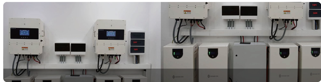
Application: Inverter -- Mars-14G1-LE Battery -- MOONI6-G Time: May, 2023 Address: Iraq Capacity: 14kW*2pcs/16kWh*4pcs
